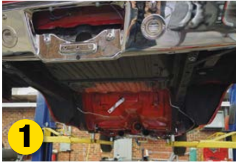
1 Disassemble the car, removing the rear axle, springs, mounts, and shocks. Also remove the fuel tank and filler tube.
