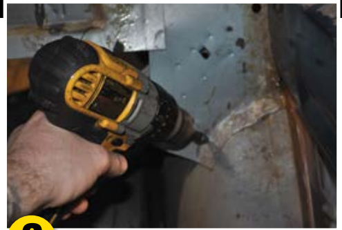
3 Drill out the spot welds holding the package tray bracket to the inner wheelhouse.
