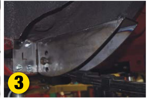
3 Carefully cut the frame rail, locate and tack weld. Mockup leaf springs in the front spring bucket. Confirm springs align with the rear frame rails.
