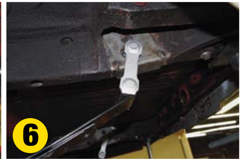
6 Fully weld the new rear spring hanger mounts (shown tacked in place).
