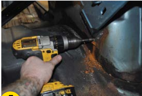
4 Drill out the spot welds holding the trunk hinge bracket to the inner wheelhouse.
