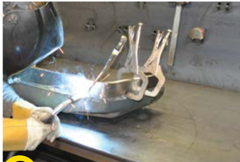
8 Once the inner wheelhouse is removed, weld the wheel tub filler in place.
